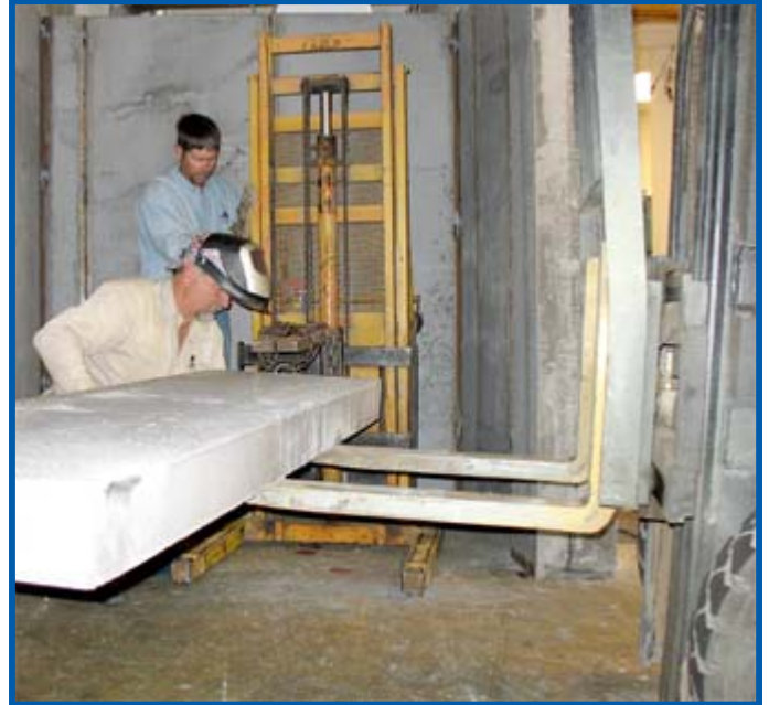
CEILING PANEL GOES UP — Two lifts are employed to put panels into place. The 8'X30" concrete and steel panels weigh more than 3,000 pounds.
