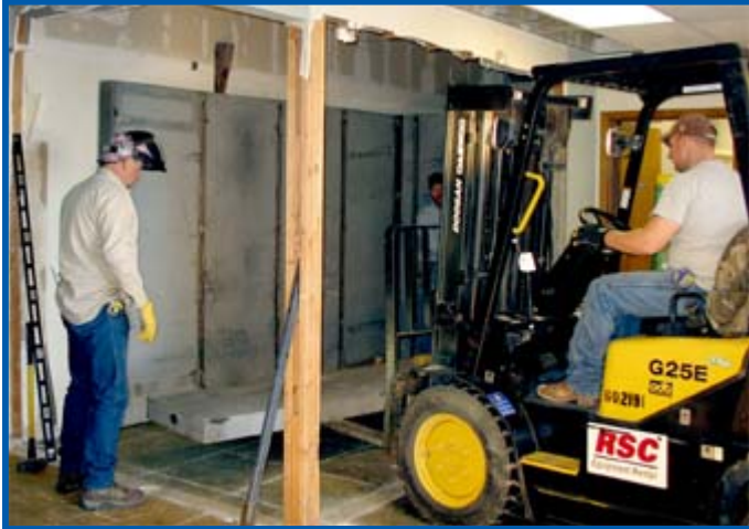
THE FITTING BEGINS — Workmen move heavy, concrete and steel panels into place before they are welded together to form solid ceiling and walls.
