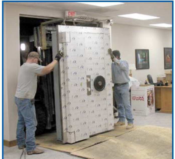
HEAVY LOAD — Two workmen and a forklift move the vault door, weighing more than 4,000 pounds, through the office front entrance. Entrance panels and the front door had to be removed completely prior to the vault installation.
