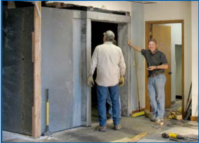
READY FOR THE DOOR — Jerry Merrill, CEFCU President/CEO, confers with the crew foreman when basic construction is complete.
